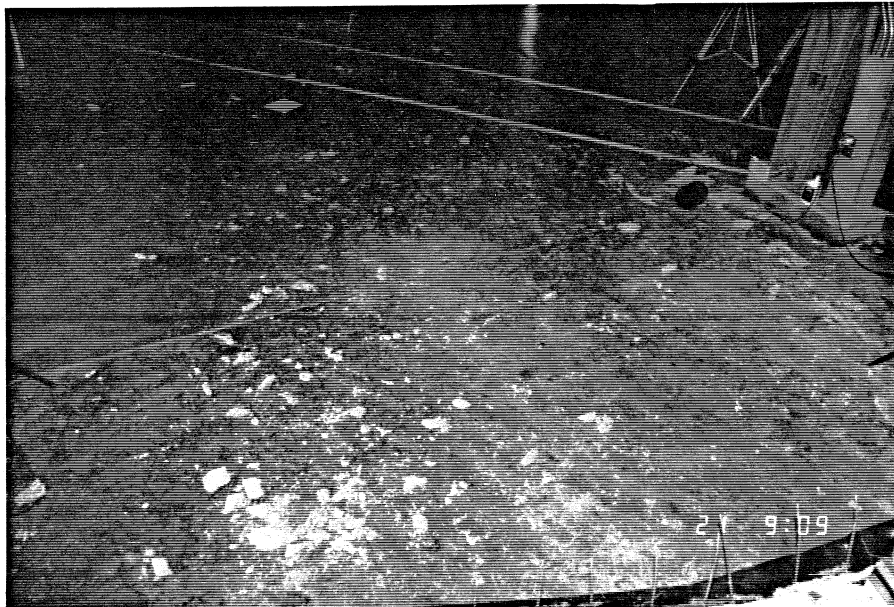
Figure 5.7 Concrete Fragments in Front of the Web
