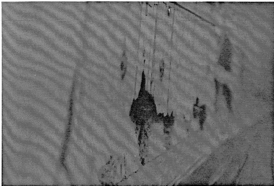
Figure 5.20 Crack Pattern of Web BC
